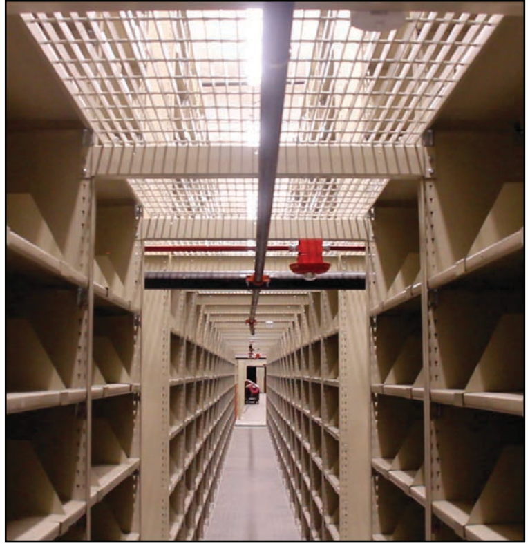
2-Story Catwalk System & Fire Suppression
